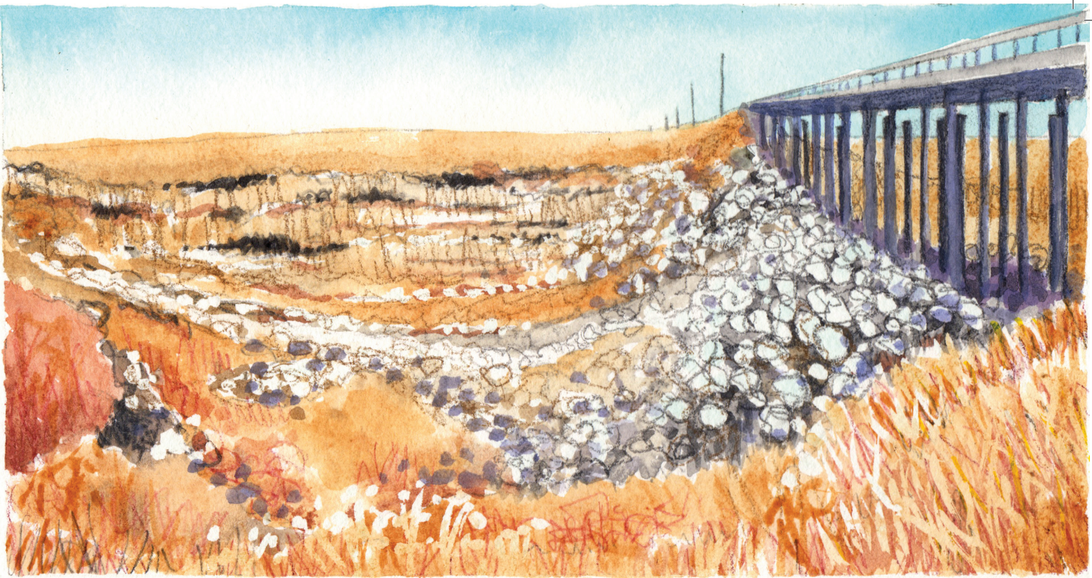
On the west side of the Valley, pilings have pulled away from this bridge due to land subsidence caused by severe groundwater pumping
