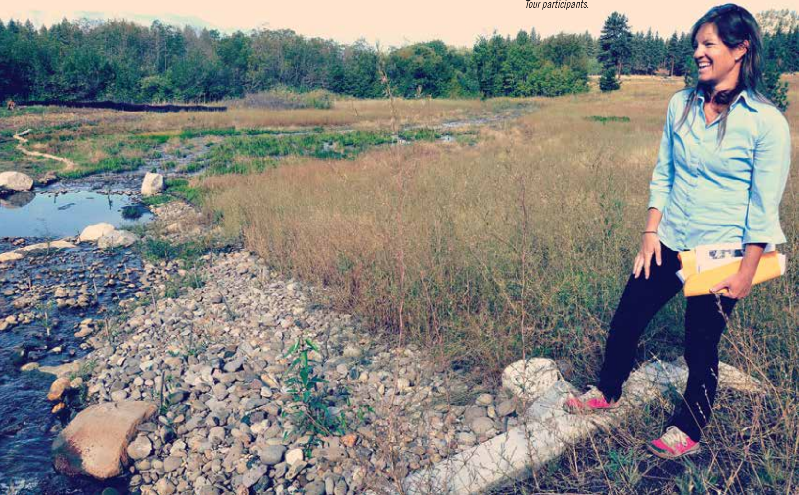
Meghan Kelly, senior project engineer/district manager with the Nevada Tahoe Conservation District, explained the Burke Creek Restoration Project to our Headwaters Tour participants.
