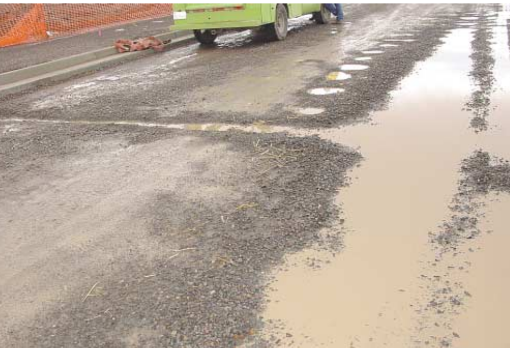
Wildcat Boulevard in Rocklin, Calif. shows uncontained, untreated runoff at development site before improvements.
