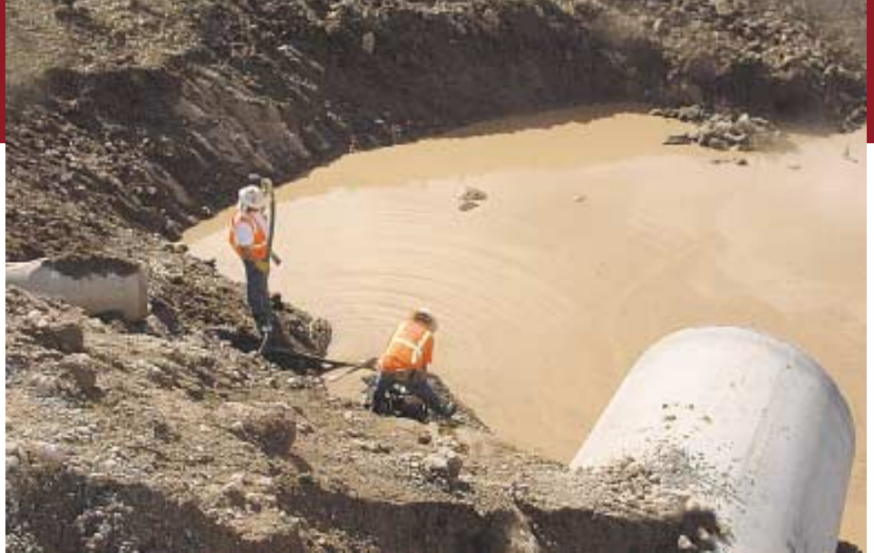
Before improvements, sediment-laden stormwater runs into detention area.
