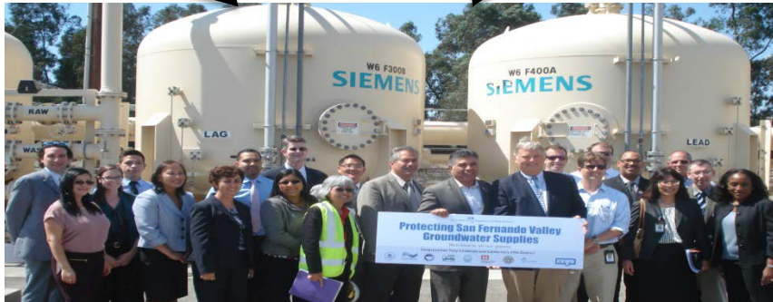
SF Groundwater Basin Remediation
