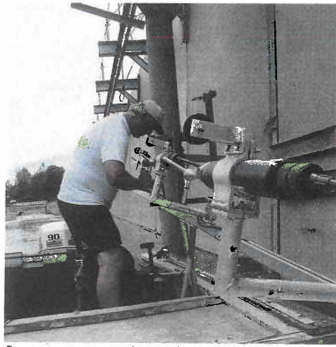
Preparing to mount three velocity probes on a screen sweep
