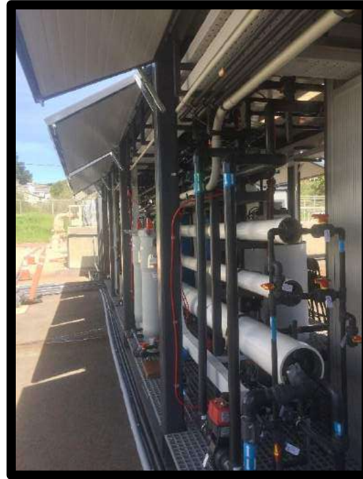
Reverse Osmosis (IDE)
