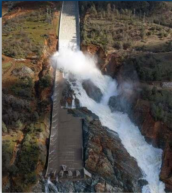
DWR's Oroville Spillway
